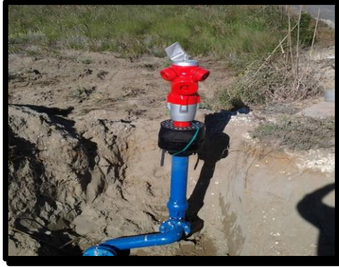
Figure VI-12 : Poteau d'incendie (Source : https://www.alertincendie.fr/details-installation+et+maintenance+des+poteaux+incendie-45.html )
