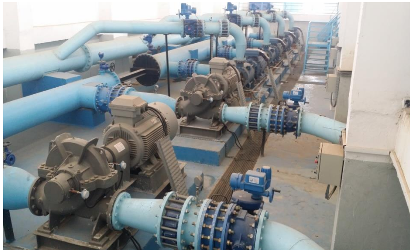
Figure III.7 : station pompage de BENI TAMOU
