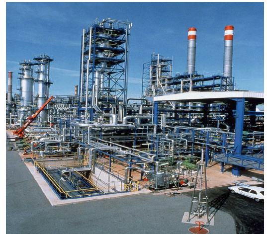
Figure .II.3: Raffinerie de Hassi Messaoud.
