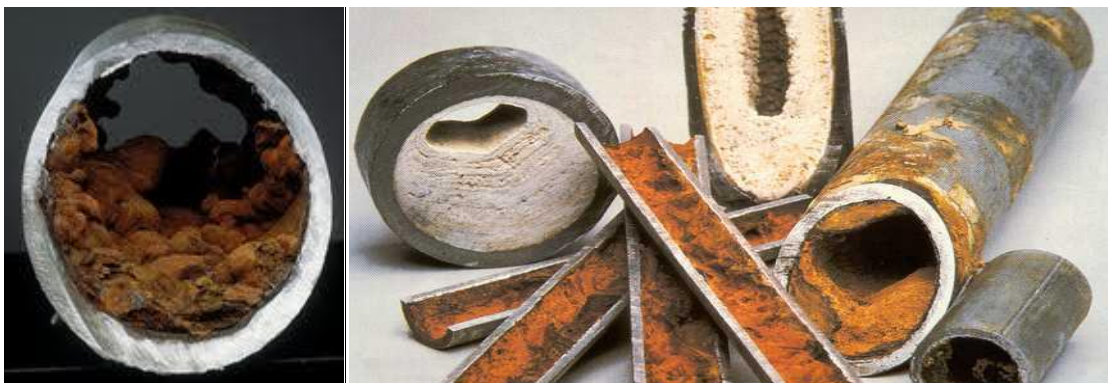
Figure VII.13 : La corrosion interne
