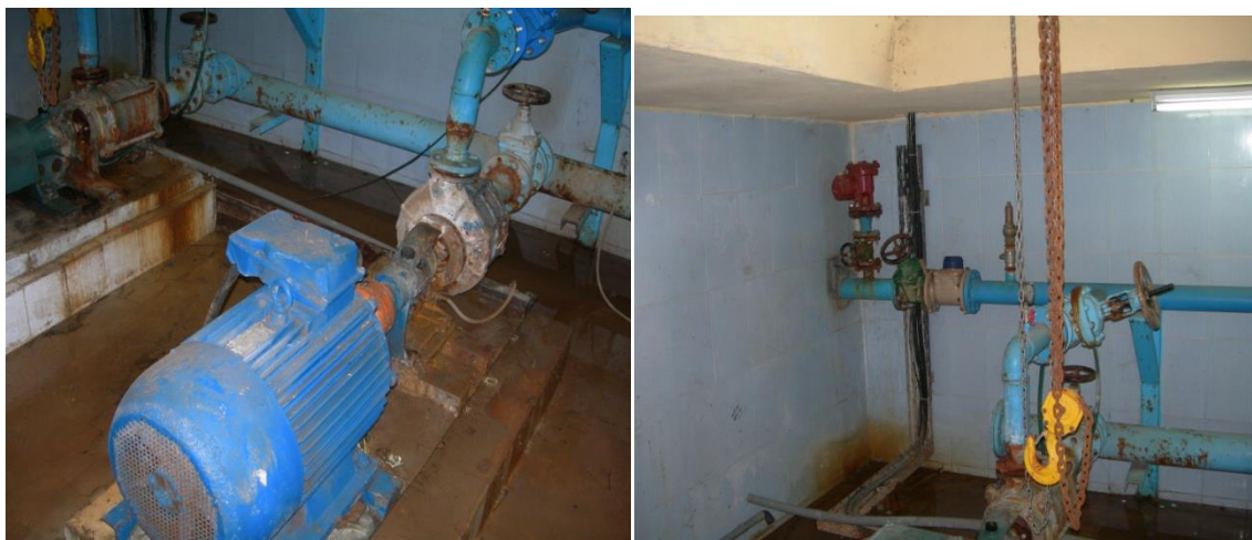
Figure II-8: Station de pompage du Douar Boucetta.
