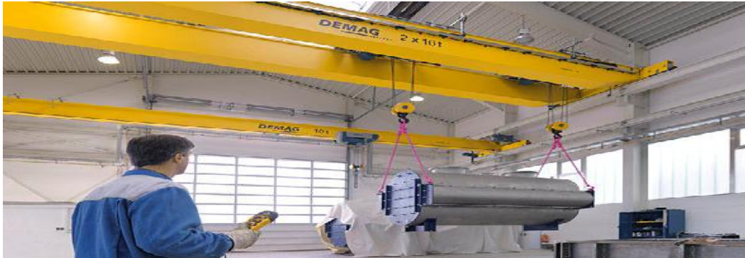
Figure V.14. Le pont roulant source (DHW, subdivision, Oued Zenati)
