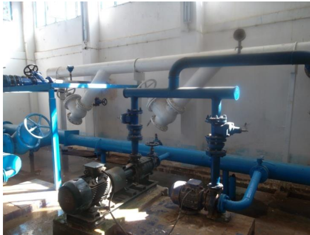
Figure 13 : Photo de la station de pompage Bakora
