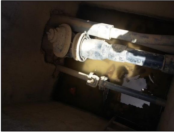
Figure III.27 : Vannes de distribution R200.
