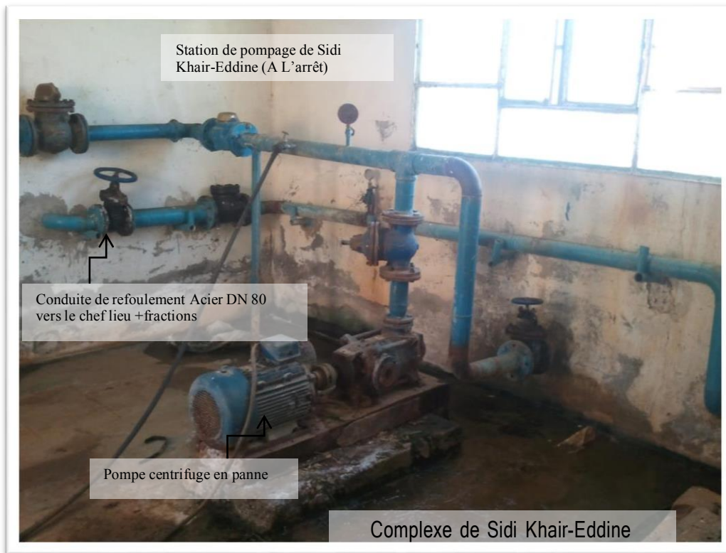
Figure I.9 : Station de pompage de station de Sidi Khair-Eddine
