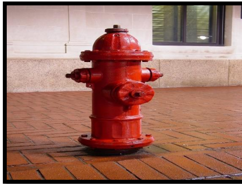
Figure VII.8: Fire hydrants and fire poles .
