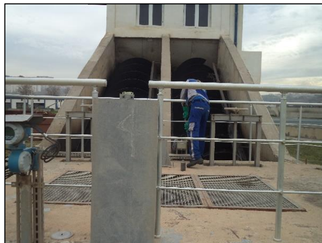
Figure III.12 : Photo de vis recirculation tranche 2 (Source : STEP de Beni Messous)
