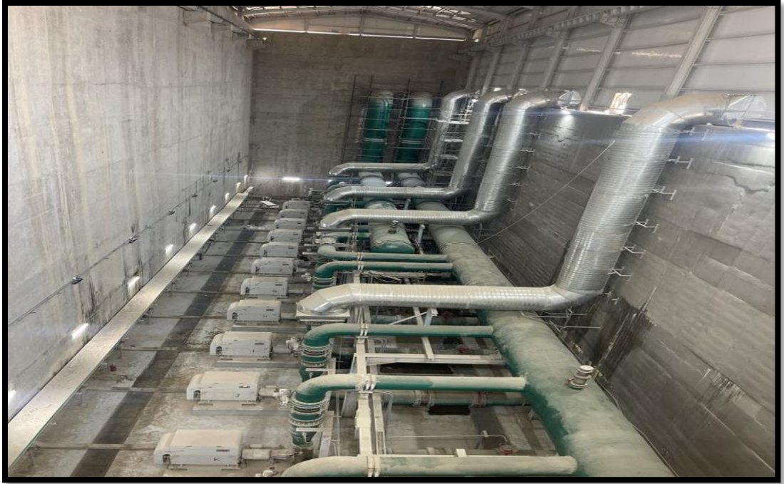
Figure III.10 – Les pompes de captages
