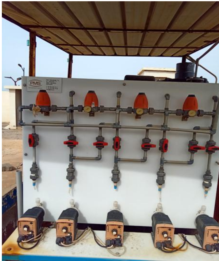
Figure III.11 : 4 Pompes doseuses + 1 secours
