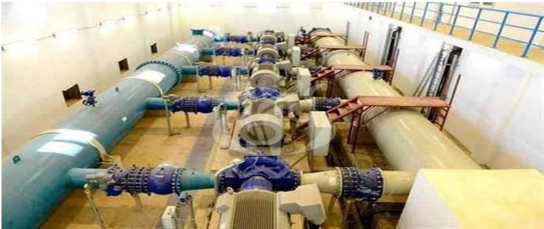
Figure III.22 : station de pompage (source aps.dz)
