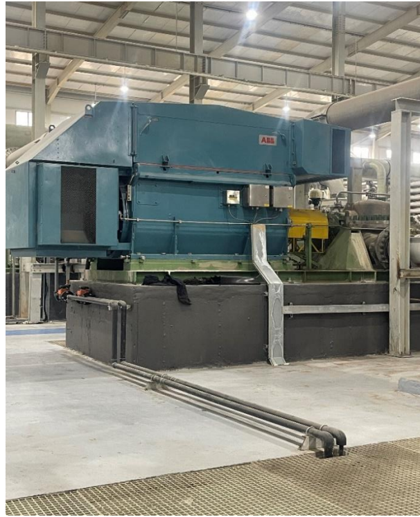
Figure III. 9 : pompe haute pression
