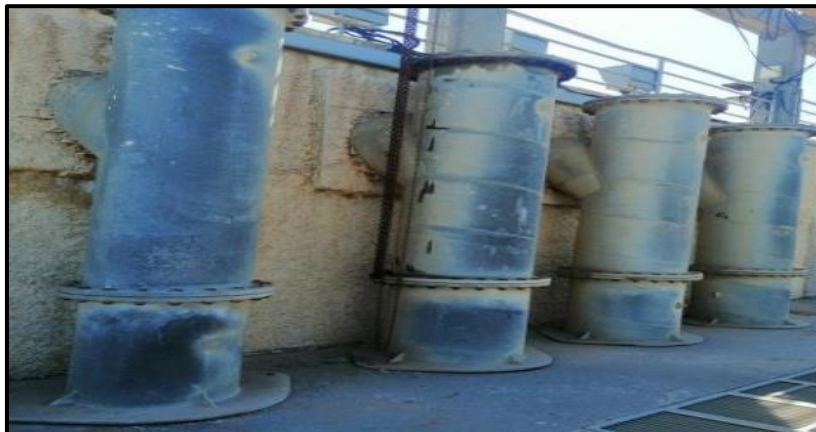
Photo II. 2 : la station de relevage
