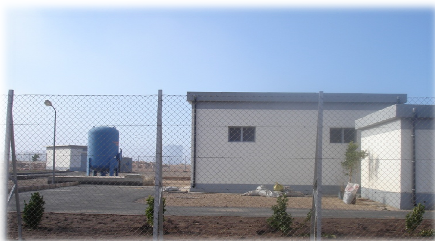
Figure 2.3 : La station de relevage
