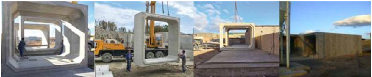
Figure VII.8 : photo de calque dalot
