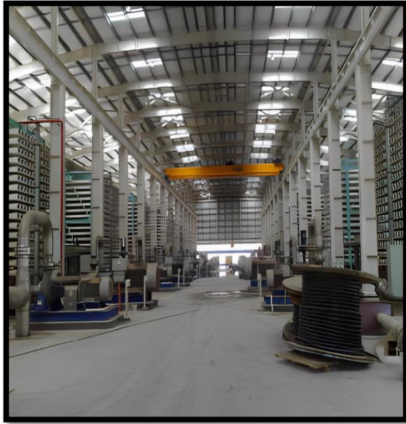
Figure II.9: Station de dessalement (SOUK THLATHA)
