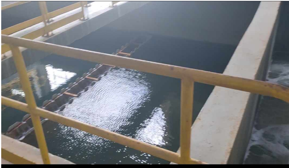
FIGURE 3.11 – Decanteur station corso
