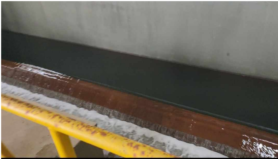
FIGURE 3.10 – Bassin de floculation station corso
