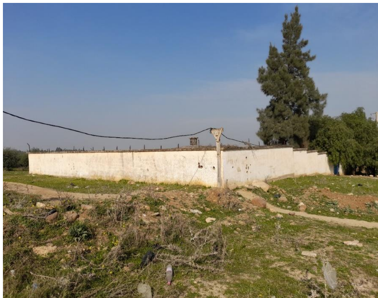
Figure III-5 : station de pompage
