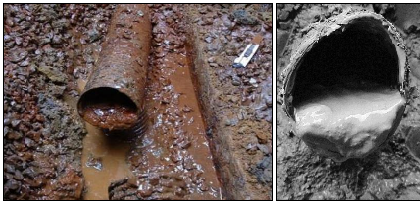
Figure VI.1: Clogging due to mineral deposit
