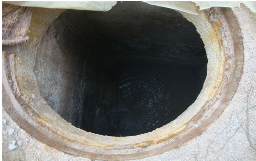
Figure II.8 : regard sans tampon
