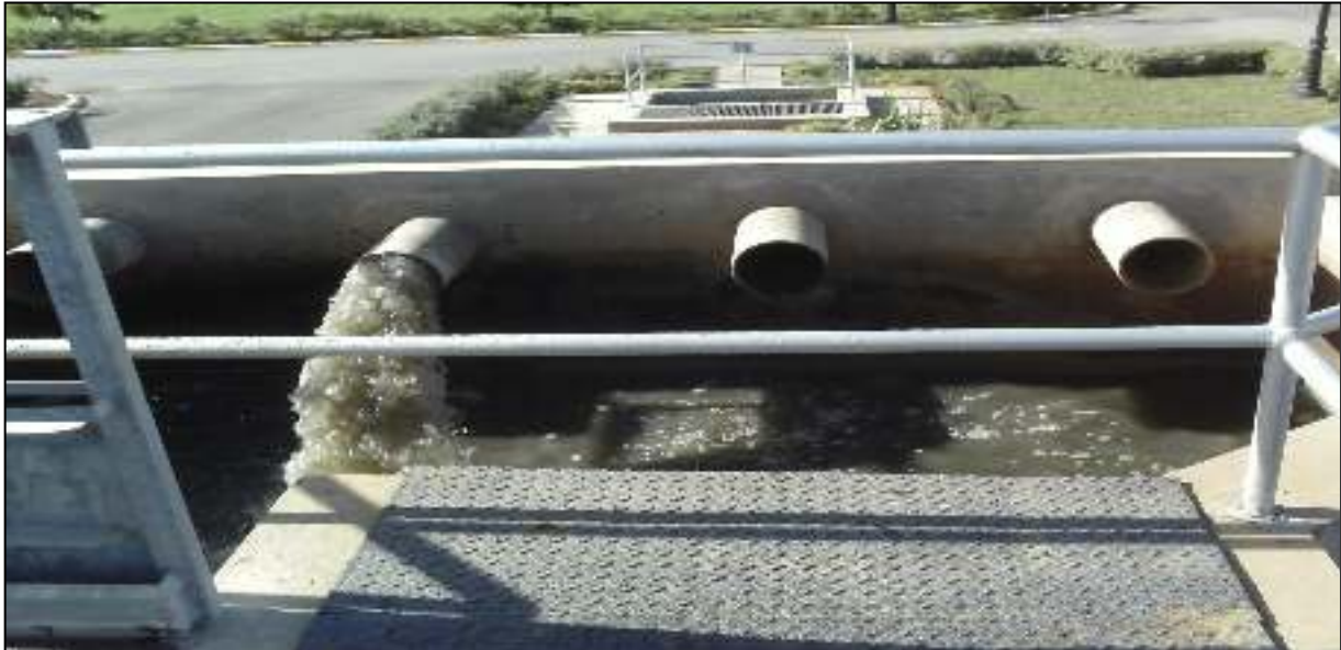
Figure II.5 : Station de relevage.
