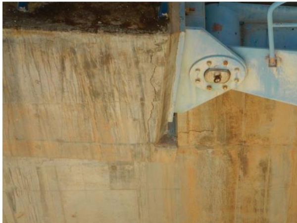
Figure III.28: Fissure sur support
