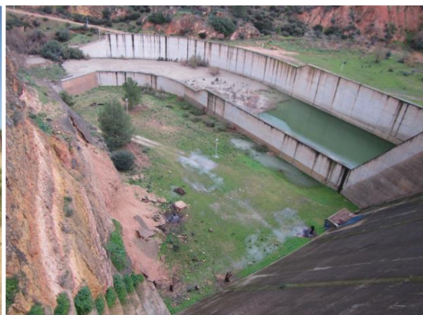
Figure III.34: Saturation du remblai aval non drainant
