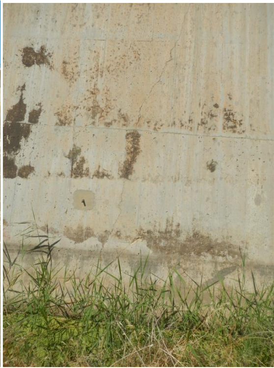
Figure III.13: Légère fissure de peau (rive droite)
