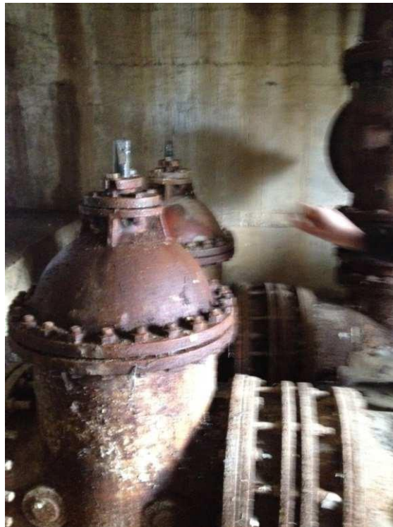
Figure II.24: Vannes de garde (ISL, 2015)
