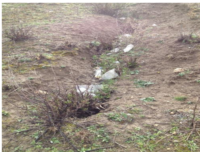
Figure II.8: Ravine sur talus aval (ISL, 2015)
