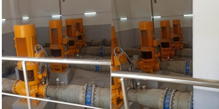
Figure IV- 6 Station de relevage
