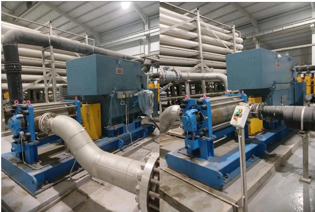
Figure IV- 15 Pompe haute pression HPRO
