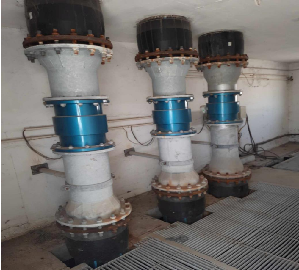
Figure 5: Pompes de relevage
