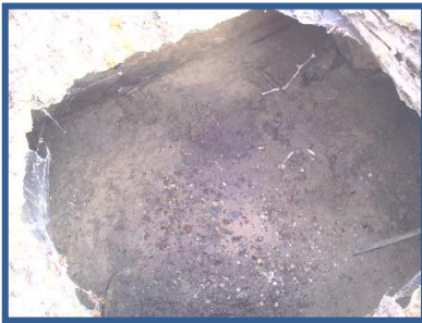
Figure 1. Regard de visite
