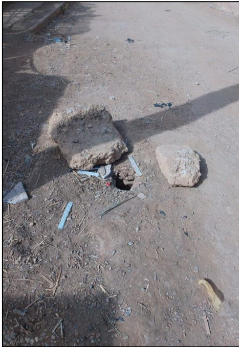
Figure III.2 Absence du tampon.
