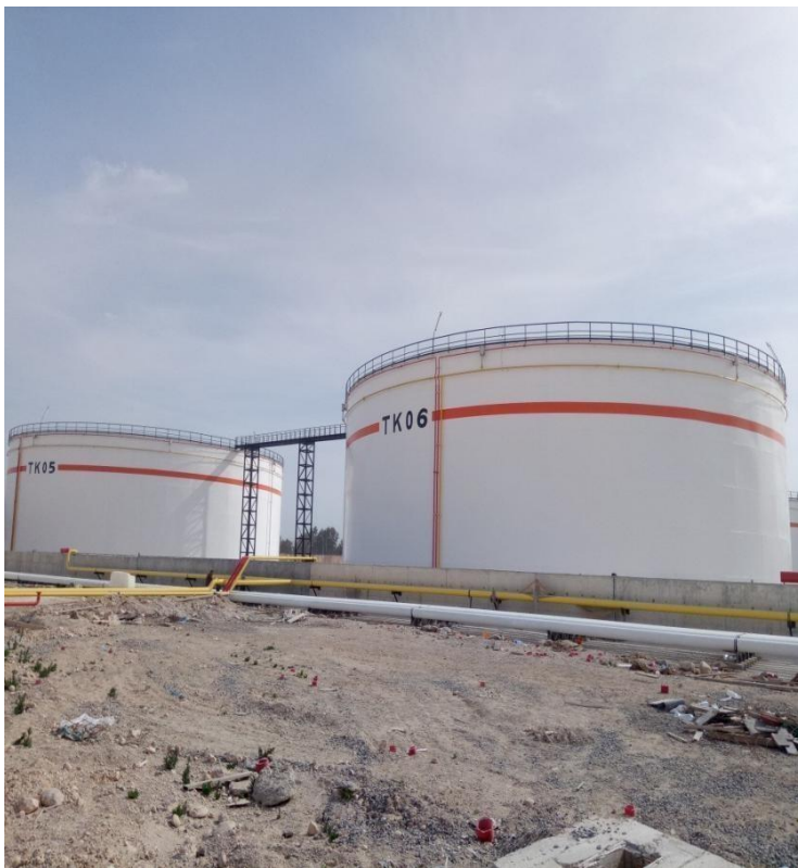
Figure 2: Bac de Gasoil 25000 m 3 (4)
