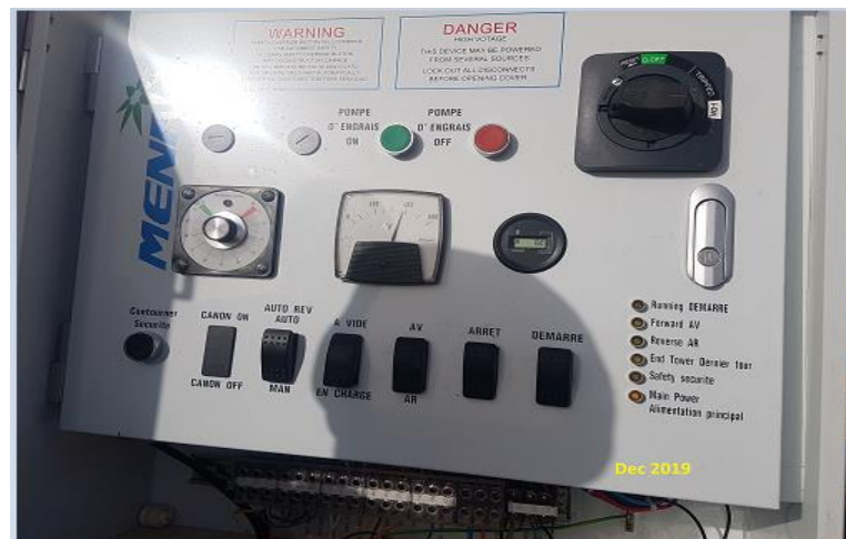
Figure V.6 : Armoire de commande, Photo COSIDER.
