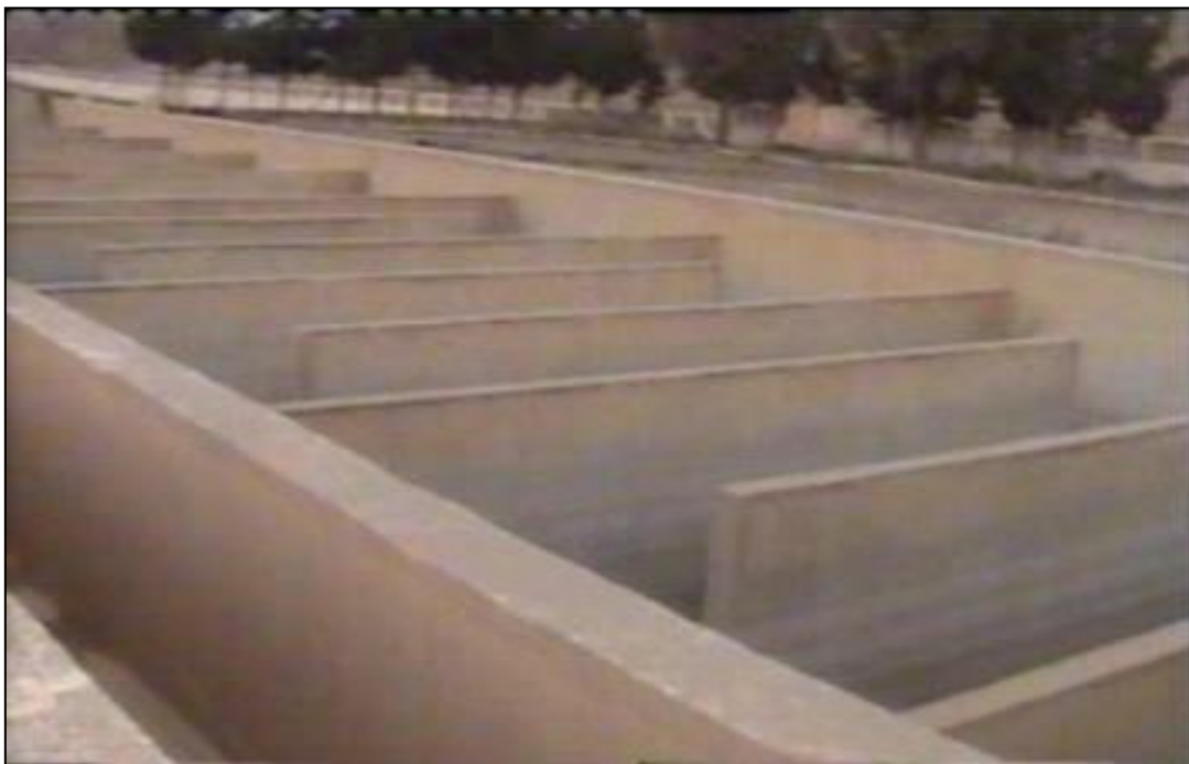
Figure II.14 : Bassin de chloration
